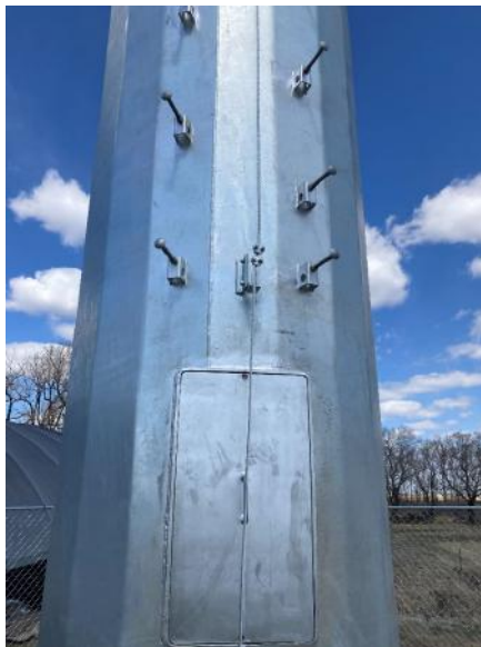
Pole Climbing Pegs and Safety Cable
