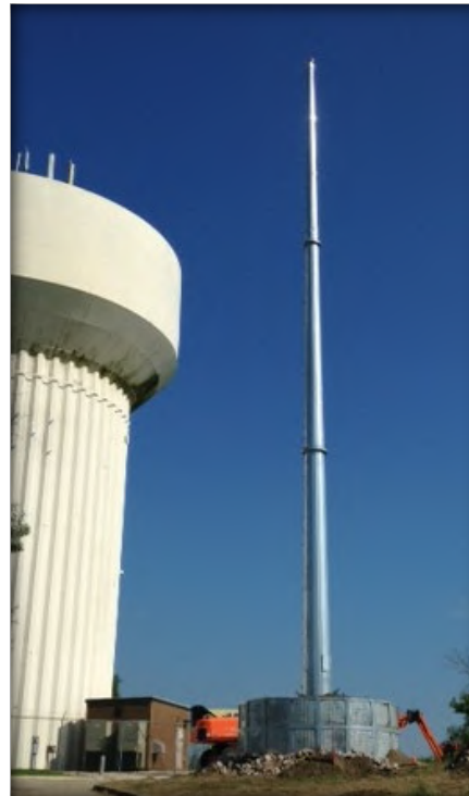
AFS 1500 foundation & 100' pole installed supporting 2-3 carriers
