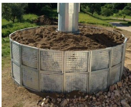
Foundation with ballast
