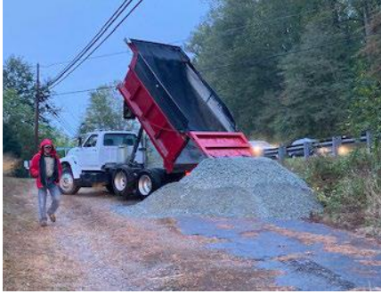
Area used to stage materials for later transport across bridge to job site
