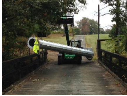
System brought section by section to the site over 8T max weight bridge
