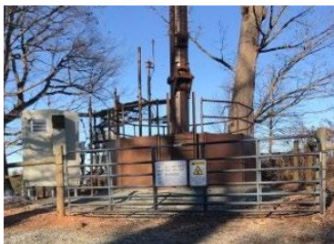
Foundation with guard rail, System painted per customer's request
