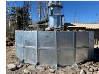
Foundation with ballast
