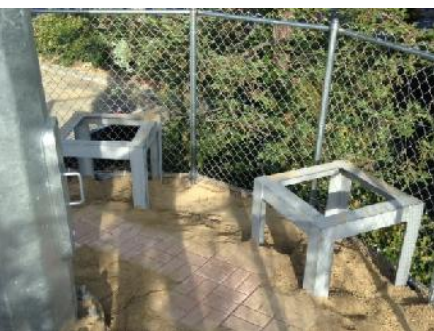
Top of cabinet holders inside the foundation
