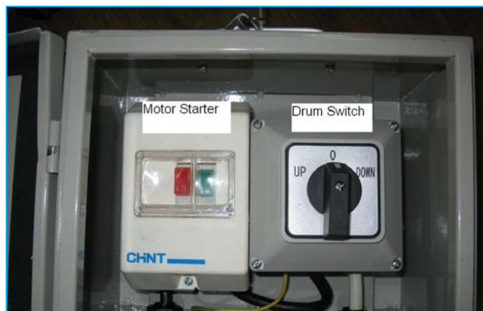
Figure 15 Control box interior
