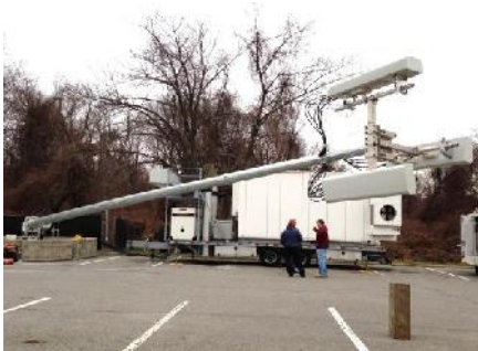
Antennas installed on pole
