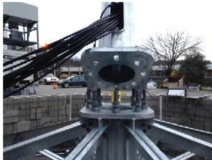
Electric wires through hand hole
