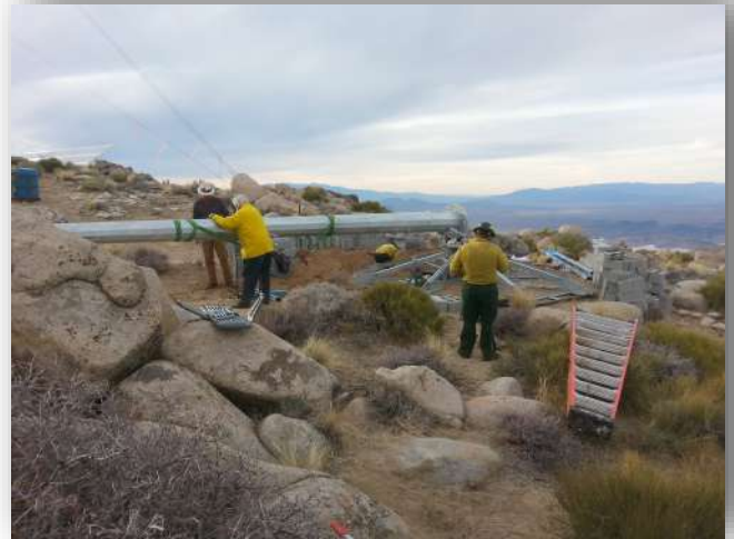
Tower pieces were picked and placed using a portable tripod rigging system.
